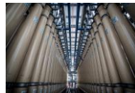
Keppel Seghers Ulu Pandan NEWater Plant
