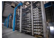
SingSpring Desalination Plant
