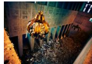
Keppel Seghers Tuas WTE Plant
